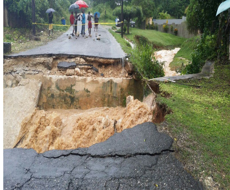
Flood damaged road in St Ann, Jamaica. Credit: National Works Agency (NWA) Jamaica
